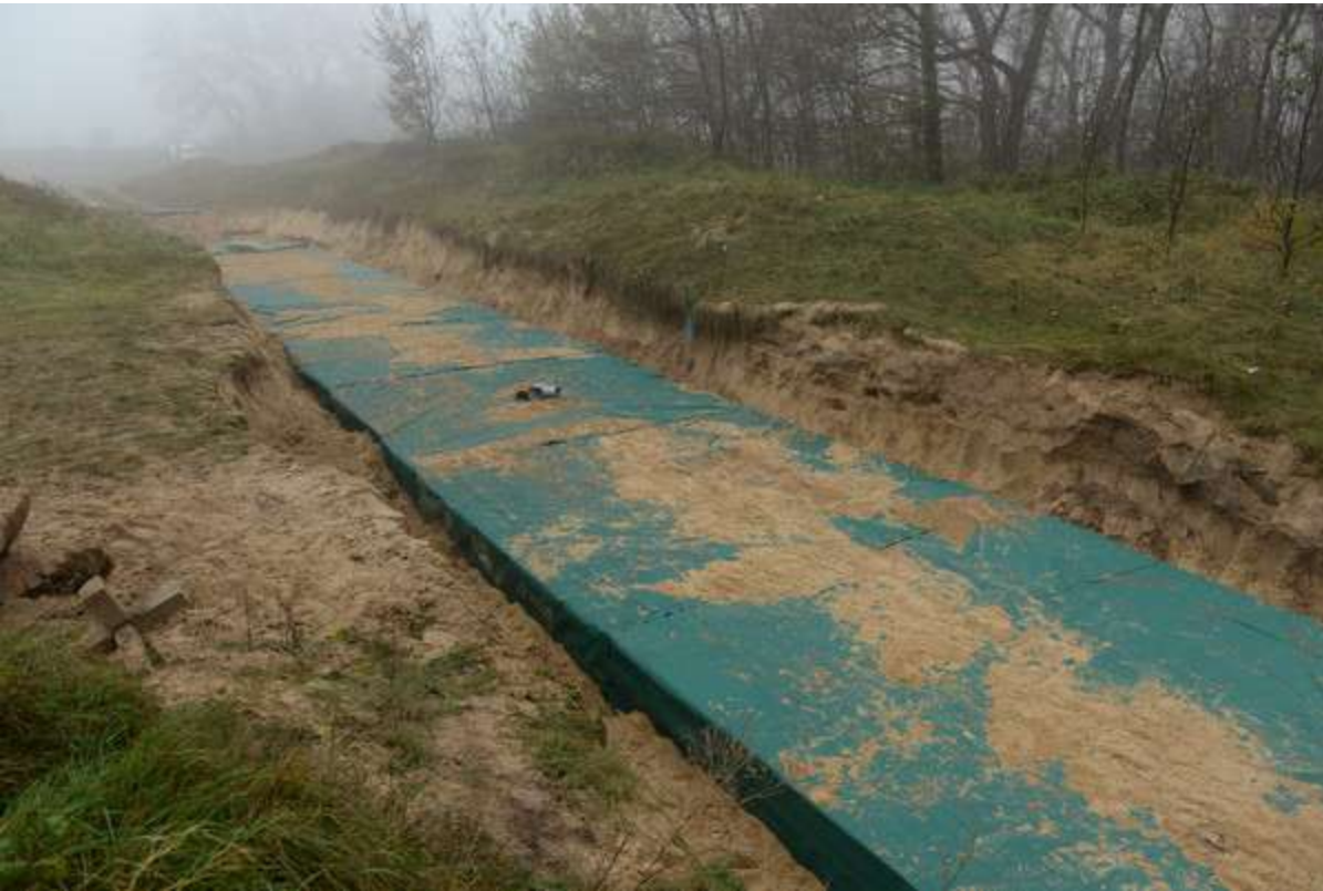
Infiltration was enhanced by implementation of 'subterranean infiltration' (since November 2014)
