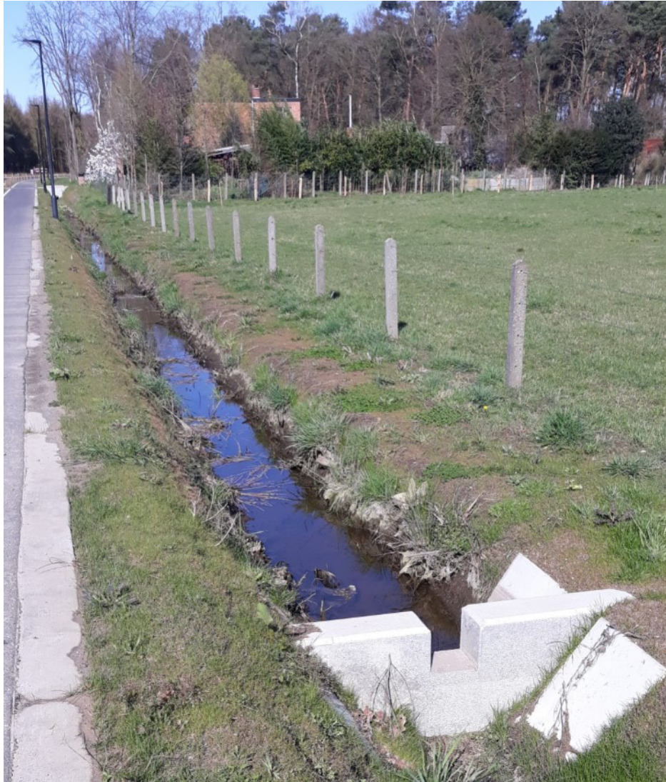
Figure 16: Creating compartments in sloping ditches for storm water drainage enable slow infiltration and groundwater recharge. Without these weirs, the water would be drained too quickly to infiltrate.
